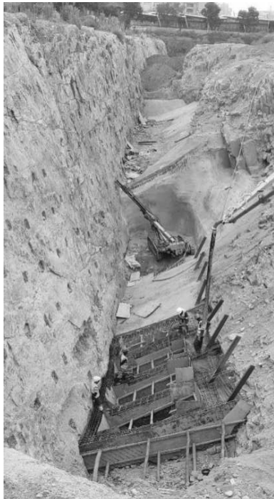
Figure 10. Temporary lateral support to facilitate safe construction of the mid-span bridge deck
