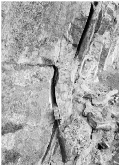
Figure 7. Joint widening in the hanging wall during excavation
