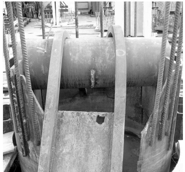
Figure 1. Failure of steel pile connection (right steel strap)
