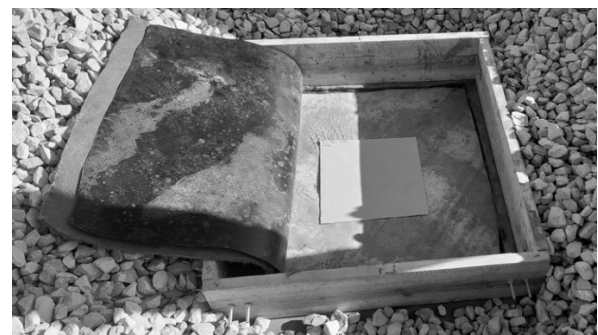
Figure 2. Metal foil sheet placed on compacted clay layer with geomembrane temporarily folded away
