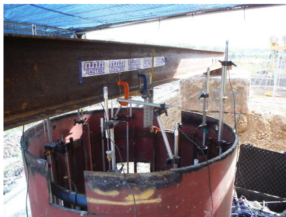
Figure 6 Instruments and reference beam over the test pile head
