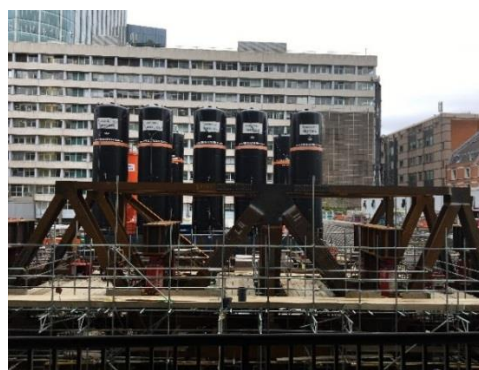
Figure 4: Test pile reaction frame with bentonite silos in the background (also used as ballast during the test)
