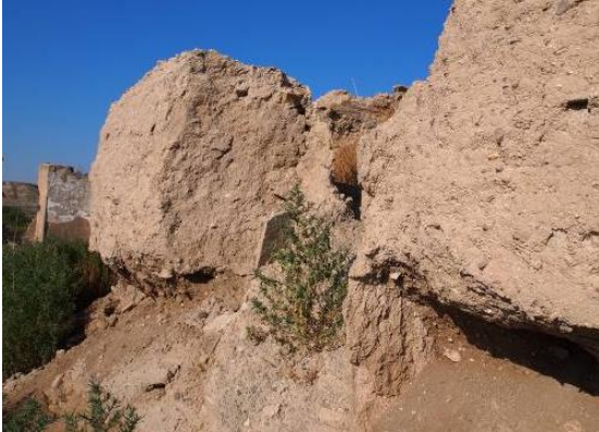
Figure 2: Severe coving of wall at abandoned monastery ruin, Mulzalcorag, near Agon village.
