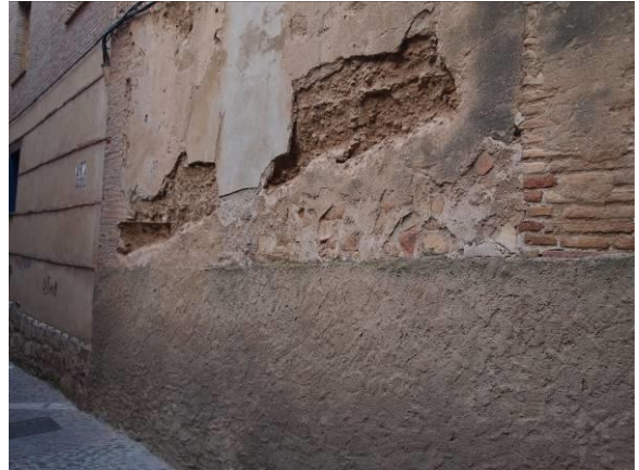
Figure 1: Rising damp and delamination of cement render exposing the RE beneath, Tarazona city.
