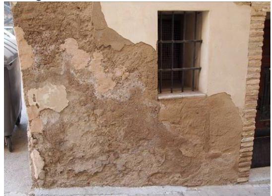
Figure 4: Surface delamination due to rising damp with salts efflorescence, Borja.
