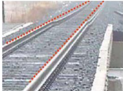
Figure 2. Unlevelled track at a track-bridge approach.
