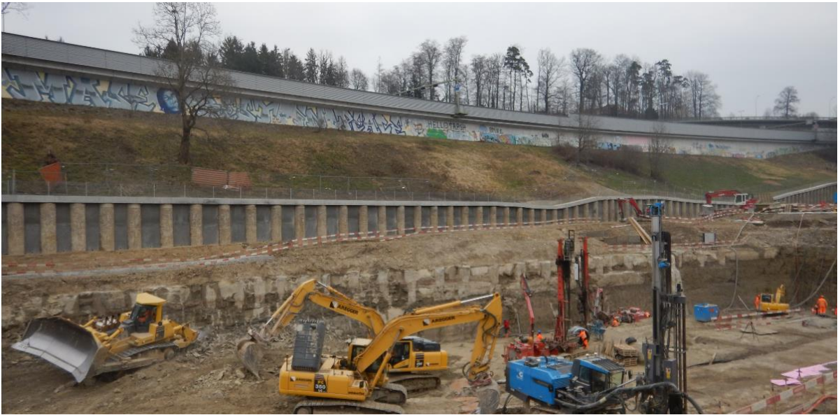
Figure 9. Finished upper (permanent) and lower (temporary) pile wall beneath the motorway embankment
