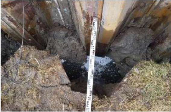
Figure 16. Gapping behind sheet pile wall AZ26
