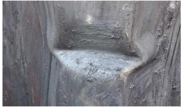
Figure 14. Excavated GU8N-rev with local buckling
