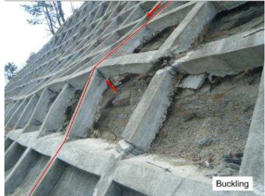
Figure 5: Collapse of shotcrete grating crib work in Kuji City after the earthquake. Buckling and shearing of the concrete ribs are observed.
