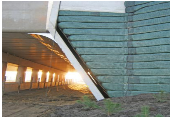
Figure 7. Executed overstep GRS Wall in the function as bridge approach and earth pressure relief to protect slender concrete wing walls of an ecoduct
