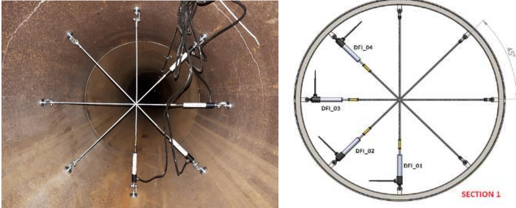
Figure 3 - Position of numbered sensors inside a sensor-equipped section of the micro-tunnel and corresponding photo.
