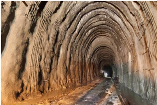
Figure 16. Sprayed concrete reinforced ribs under construction. Bending of the tunnel alignment ahead.
