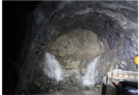
Figure 4. Inflow of water from fault plane 5m ahead.
