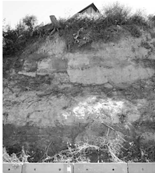
Figure 8. Roots and granular soils at the crest.
