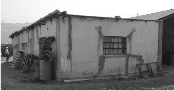
Figure 6. Cracked buildings on site showing evidence of expansive clays
