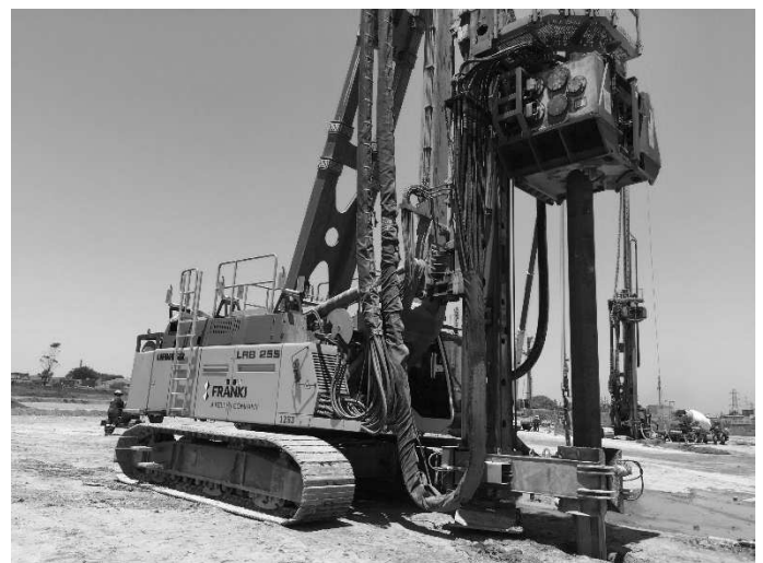
Figure 2. Liebherr LRB 255 crawler rigs equipped with ring vibrators for driving steel tubes
