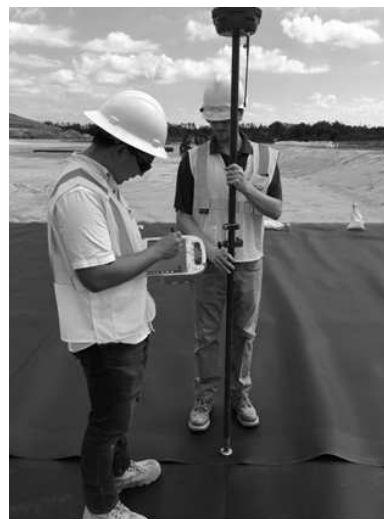
Figure 10. Photo of GPS location of a “T” joint, courtesy of COMANCO
