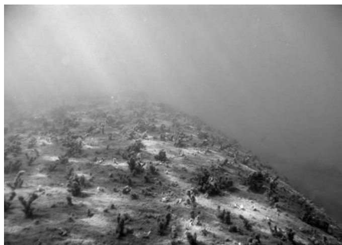
Figure 5. Geotextile tube surface 13 months after installation (Aminti 2010)
