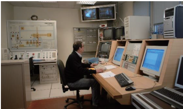
Fig.3. The former control room (†Gérard Rault circa 2011)
