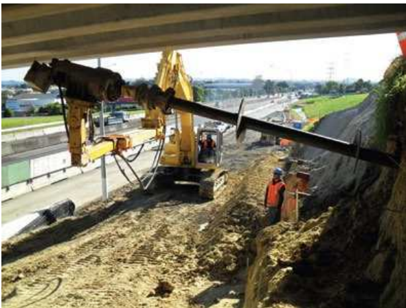
Figure 1. a) Screw Piles used for Re-levelling and Strengthening existing Foundations after Quake Damage b) Screw Piles used for Anchoring (IPENZ, 2015)
