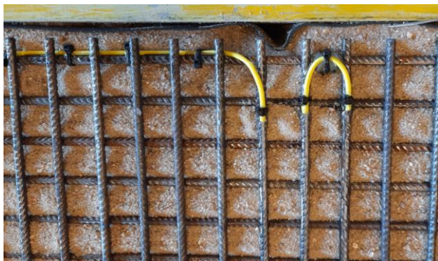
Figure 3. Fibre optic sensors measuring steel reinforcement strain (yellow tubes were used for protection of the acrylate-coated fibres in sections where fibres needed to be bent).
