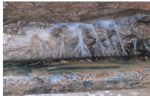
Figure 2 Erosion and void formation around breached pipe (water matters UK.2013).
