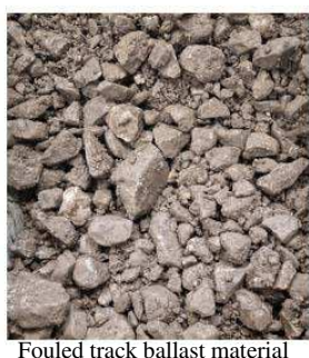
Fouled track ballast material
