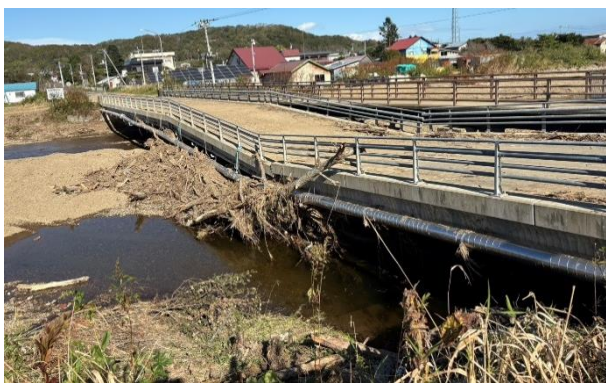
Figure 1. Case study of bridge damage caused by trapped driftwood.
