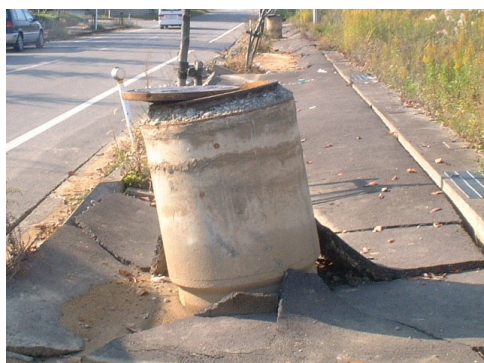
Figure 2. An example of manhole uplift resulting from the 2004 Niigata Chuetsu Earthquake.
