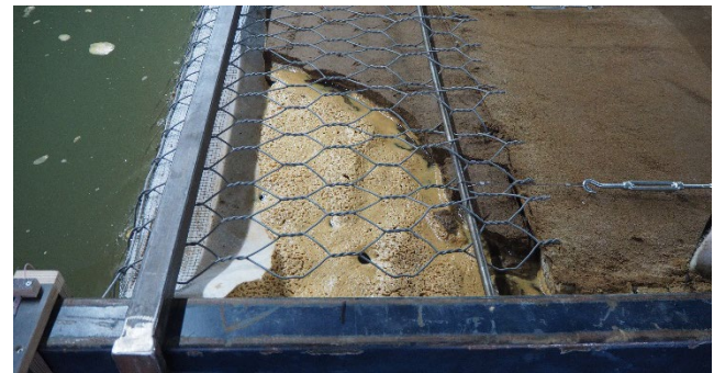
Figure 11. Visible erosion processes on the dam surface.
