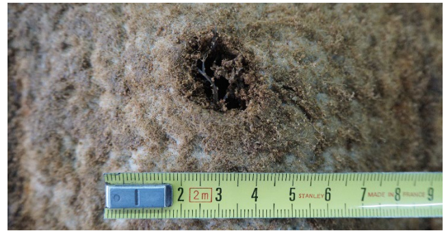
Figure 7. Artificially introduced hole in the GCL-sealing.
