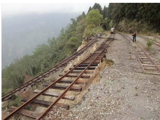
Figure 2. The scarp of the landslide that induced losses of railway foundations in Alishan Mountain.
