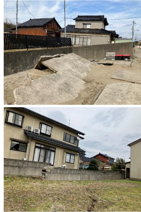
Figure 3. Damaged houses due to liquefaction-induced lateral spreading
