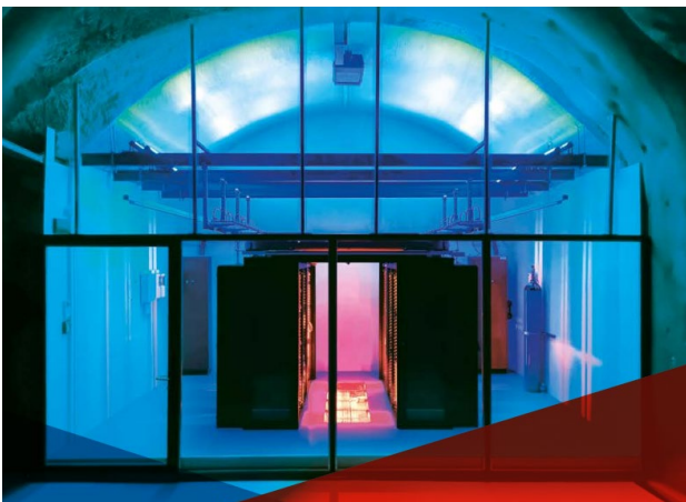
Figure 4. Photo of the Edge Computing installation
