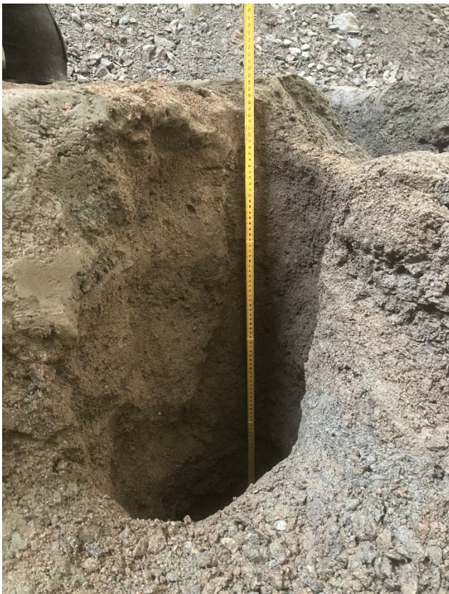
Figure 6. Eroded core soil removed, leaving the intact core soil in place during dismantling. Damage ~120 cm deep with an estimated volume of 300 litres.
