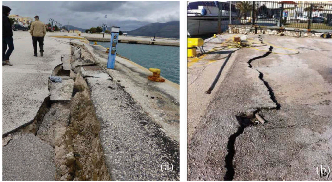
Figure 3. (a) Displacement of the quay wall in Lixouri port, across the Plaza of National Resistance following the second earthquake (GPS coordinates: 38.199444, 20.439444); (b) displacement (~16 cm) of the quay wall in Argostoli port.
