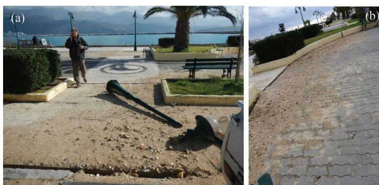
Figure 1. Examples of gravelly soil liquefaction through pavement construction joint at the port of Lixouri following the second earthquake. Note the large particle size of the ejecta (a): 38^{\circ}11'55.38''\text{N} , 20^{\circ}26'20.98''\text{E} ; (b): 38.199166 , 20.439166 .
