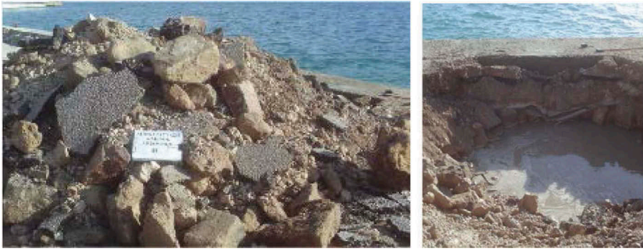
Figure 4. Views of debris excavated adjacent to the port seafront at the location where the maximum lateral displacement of the quay walls was registered in Lixouri. The large particles of the fill material is visible. (Geoconsult Ltd, 2016)
