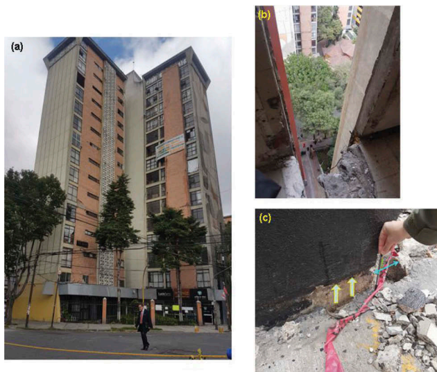
Figure 2. The Osa Mayor rocking failure: (a) plan view of the 15-floor RC double L-shaped building, (b) the opening between the two L-buildings as seen from the 11th floor, and (c) detail of the uplifted corner (with the turquoise double end arrow is noted the horizontal gap induced by the rocking motion of the building).
