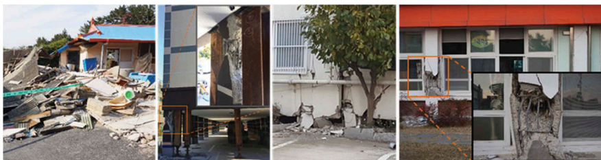
Figure 1. Examples of structural damages caused by the 2017 Pohang earthquake.
