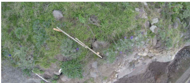
Figure 5. Typical deformation markers on the cliff edge as monitored by UAVs, combining established geotechnical monitoring tools with state-of-the-art remote sensing and survey tools. Note the large cracking of the 80m high cliff edge.
