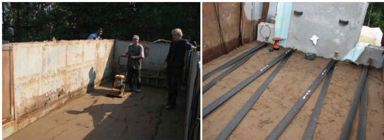
Figure 5. Compaction of soil (a) and connection of geostrips to concrete facing panels (b).
