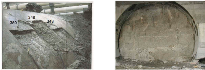
Figure 10. Photographs of the damage tunnel (rings 348 to 350) and tunnel's cut showing "light grout" tunnel filling (Salgado, 2009a, 2014)
