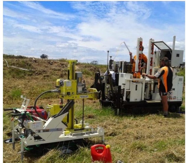
Figure 2. SDS test on the left side and small CPT rig on the right side
