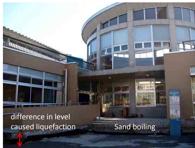
Picture 1: Liquefaction damage at Area 1
