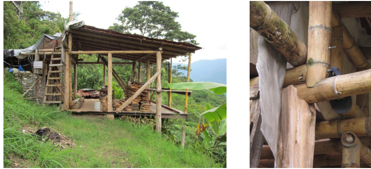
Figure 1. Bamboo-framed house under construction in Cañas (Guanacaste region), in Costa Rica, precariously adapted to a steep topography (Photos by V. López-Ausín)
