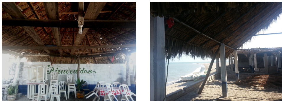
Figure 2. Left: Interior of a timber-roofed building with randomly mixed RC and timber columns and a single unreinforced masonry wall. Right: improvised wooden posts against poorly connected RC columns of the same building (Photos by S. Ortiz-Palacio)
