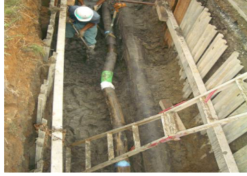
Figure 1. Upheaval buckling of 4” pipe
