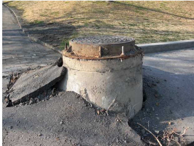
Figure 1: Manhole uplifted during the 2011 Off the Pacific Coast of Tohoku earthquake in Urayasu City.
