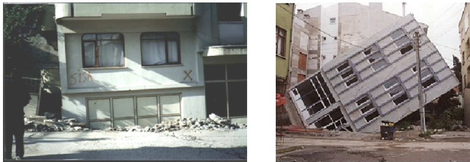
Figure 1. Liquefaction induced damage during the Kocaeli earthquake of 1999 in Turkey (adapted from Madabhushi and Haigh, 2009)
