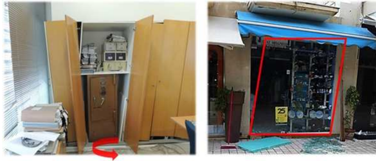
Figure 8. Nonstructural damage: Sliding and rotation of bank vault (left); glazing failure (right).
