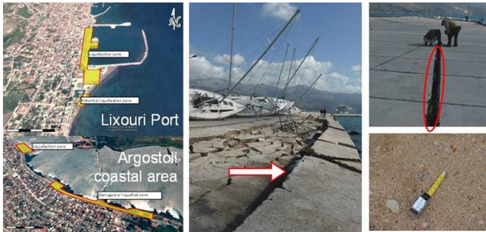
Figure 3. Liquefaction zones at two main ports of Lixouri and Argostoli (left). Lateral spread at Lixouri quay wall (middle); opening of joint at pier and evidence of gravel in ejecta (right).
