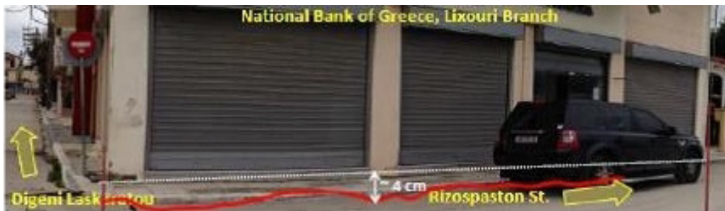
Figure 5. Settlements between the base of the National Bank Lixouri branch and sidewalk.
