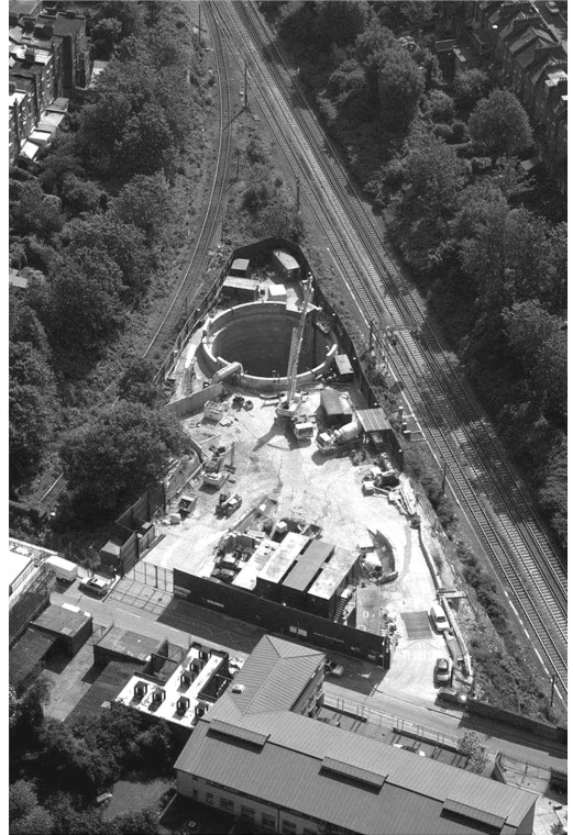
Figure 1. An example of the constraints: a shaft site located between two railway lines.
