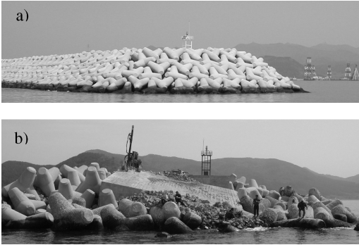
Figure 2. Effect of typhoon waves on a breakwater in Busan (typhoon Maemi, 12.9.2003): (a) before and (b) after the storm.
