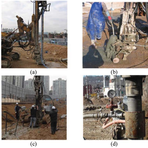
Figure 7. Procedure for installation of pressurized grouting ground anchor: (a) drilling with double casing; (b) gravitational grouting; (c) insert tendons into the borehole; and (d) pressurized grouting.
