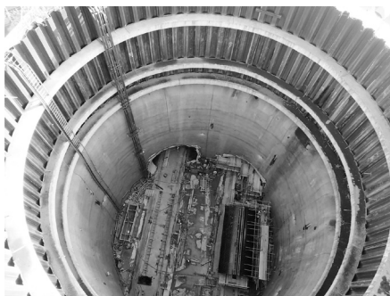
Figure 8. Crossrail's 28 m diameter, 39 m deep auxiliary shaft constructed using a combination of pre-installed sheet piles and a sprayed concrete lining.
