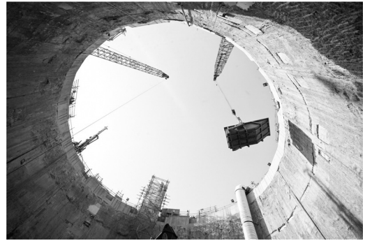
Figure 5. View from the bottom of Crossrail's 30 m diameter 44 m deep main TBM launch shaft at Limmo Peninsula.
