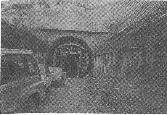
Figure 4. Formwork for the construction of the final lining entering the southern portal.
