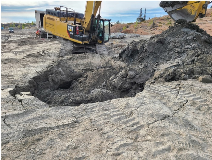
Photograph 2: Unworkable conditions prior to dewatering, sinking of equipment
