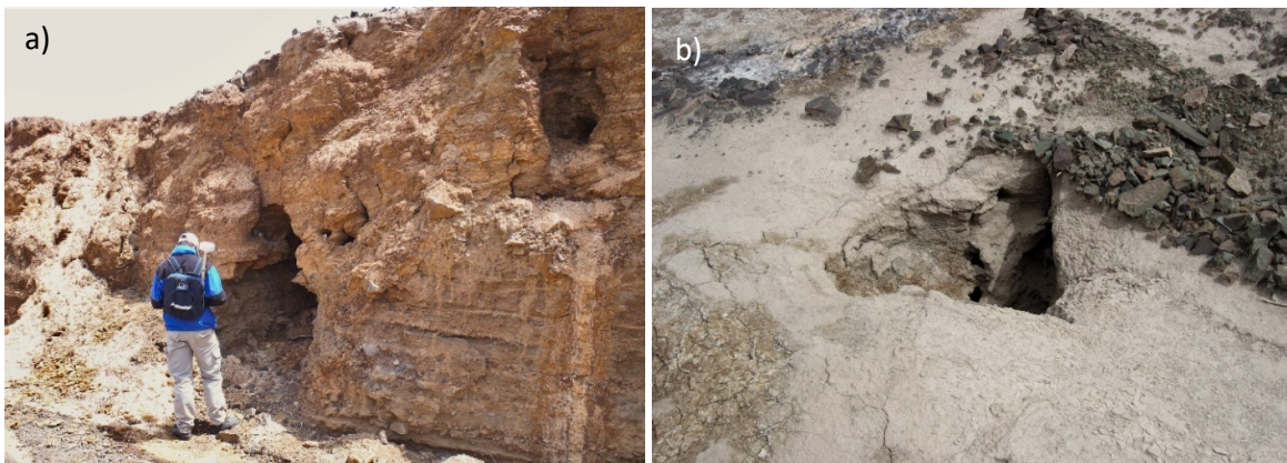
Figure 5: a) Caverns presumably formed by piping due to leaks into the decant pipe. Note bending of the strata above the cavern roof. b) Sinkhole found at the top of the tailings beach in correspondence with the caverns shown in Figure 5a.
