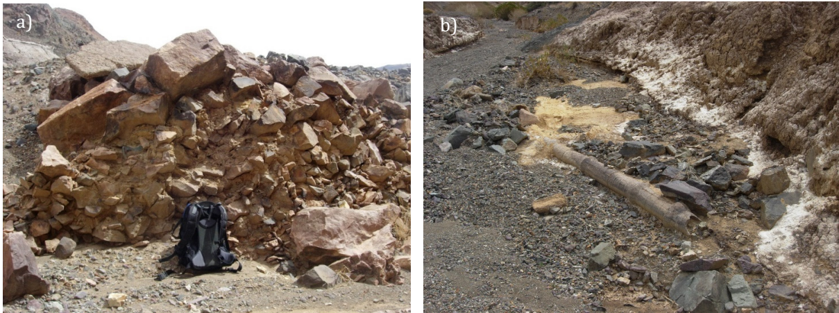
Figure 3: a) Starter dam. Note the rockfill voids invaded by tailings. b) 200 mm precast concrete pipe laid in the valley bottom as decant pipe.
